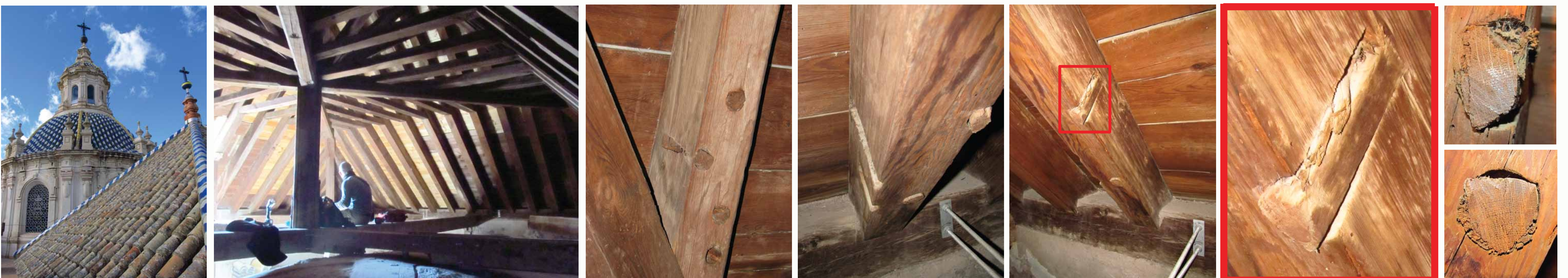
Fig. 3. Left to right: outer and inner roof of the dome above the southern transept; oak wooden pegs held by twigs in different beams. Photos: M. Domínguez Delmás and S. van Daalen.
