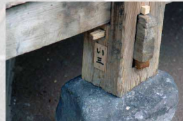
Restoration of a wooden pillar lying on a flagstone, showing details of the assembly of the old and new parts.
