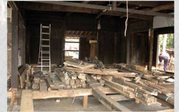
Inside view of the house during the reconstruction: The place of each part was thoroughly noted before dismantling. Floor of the main room.
